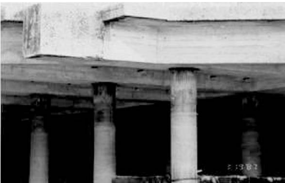
Fig. 6. Steel piles with corrosion.
